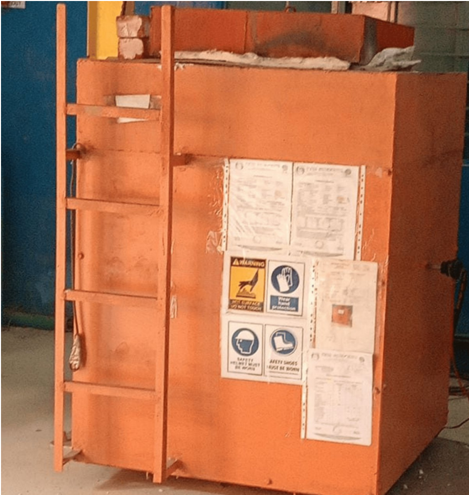
FIGURE 3: Electric furnace setup
