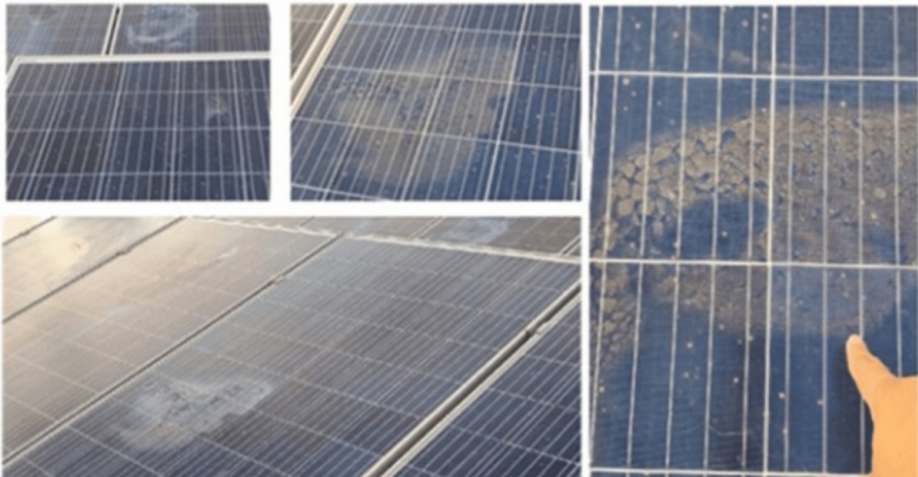
FIGURE 1: Examples of PV module failure due to hotspot on PV module PV, photovoltaic
